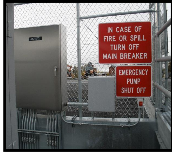
Emergency Shut-off Switch
