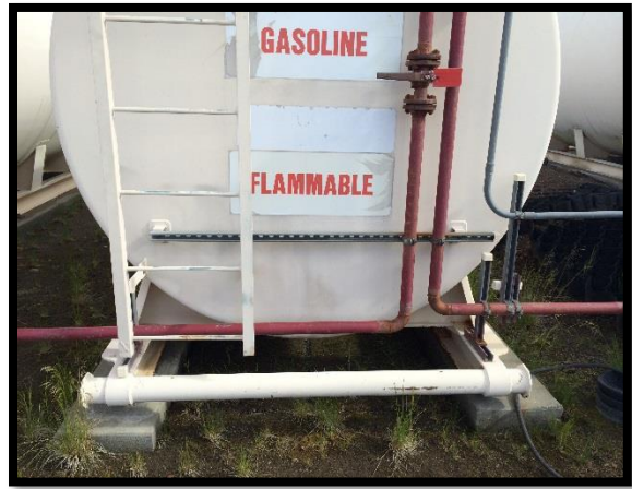
Skid Mounted Tank on a Concrete Foundation
